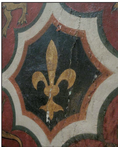
Flaking paint on the Quire panelling to the east side of the Pulpitum Arch
